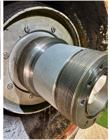
Belzona 1111 (Super Metal) was left to cure and machined to original dimensions.
