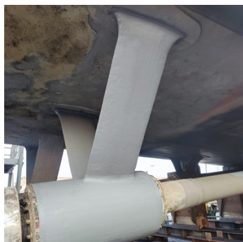
Belzona 1111 (Super Metal) was used to rebuild and fair the pitting damage on the substrate
