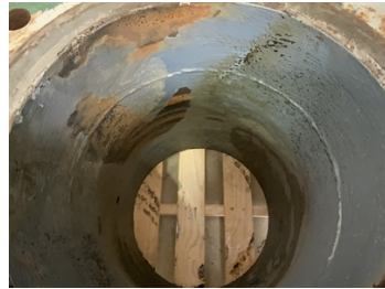
You can see the old coating had started to wear off.
