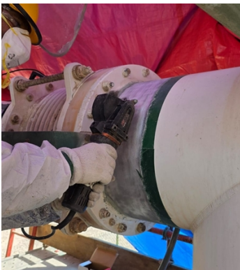
Surface preparation of bond areas in accordance to SSPC-SP 11 using MBX Bristle Blaster.
