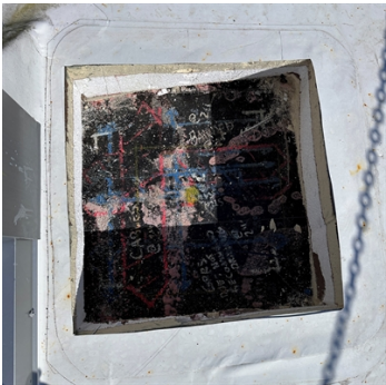
Roof surface showing interference inside roof slab
