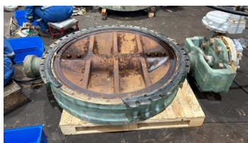
Critical erosion-corrosion damage in butterfly valves.
