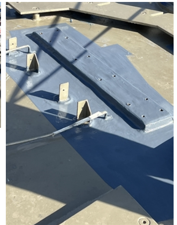
Close-up view of Belzona 1111 (Super Metal) being applied to repair pitting, followed by Belzona 1321 (Ceramic S-Metal) coating on the vessel deck
