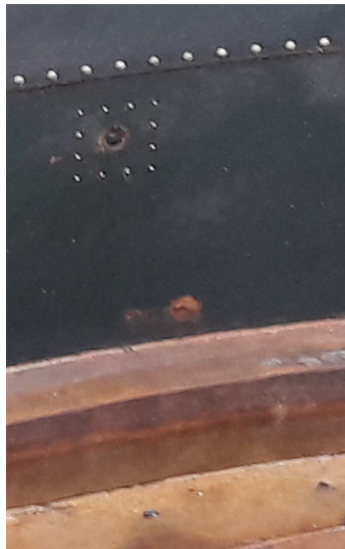
Example of defect from inside the tank
