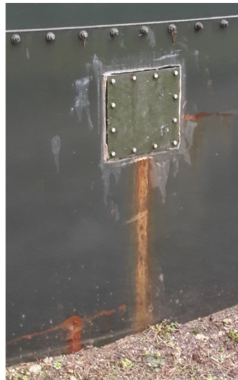
Example of defects from the external
