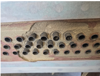
Metal loss observed on the heat exchanger tube sheet.
