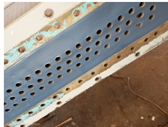
The tube sheet was rebuilt using Belzona 1111 (Super Metal) and coated with Belzona 1321 (Ceramic S-Metal).
