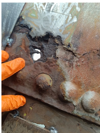
Damage to the tank
