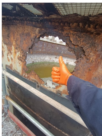
Further larger damage to the tank
