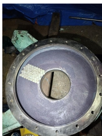
Belzona 1161 (Super UW-Metal) rebuild completed prior to installation of Belzona 9811 Alumina Tiles
