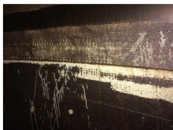
Scratch damage and wearing
