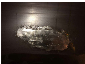
Damage to the impeller
