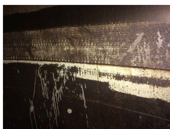
Scratch damage and wearing
