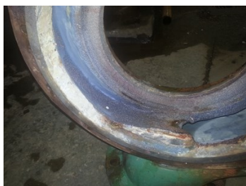
Damaged internal surface of the pump.
