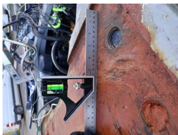
Metal loss shown on the casing
