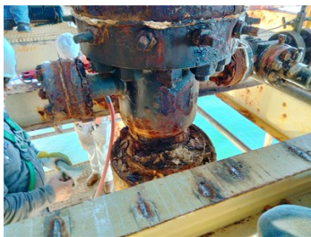
Original condition of the leaking wellhead.
