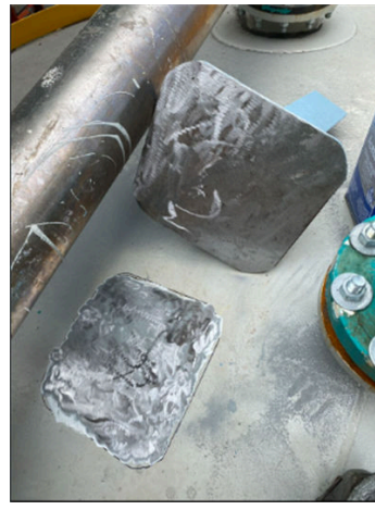
Areas on top of the tank prepared with a Bristle Blaster to remove paint.
