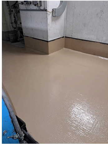
Belzona 4111 (Magma-Quartz) was used to build a cove at the joints with the perimeter walls, and overcoated with Belzona 5831 (ST-Barrier)
