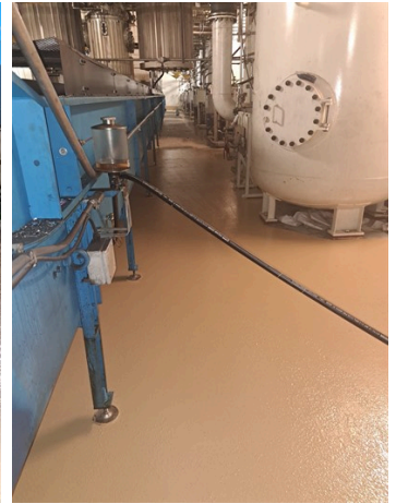
The concrete underneath the conveyor lines were protected and made safer by the repair
