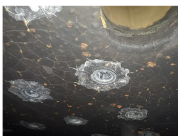
Cracking on the original rubber lining
