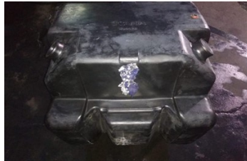
Cracked and leaking fuel tank
