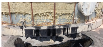
Live hydrocarbon leak.
