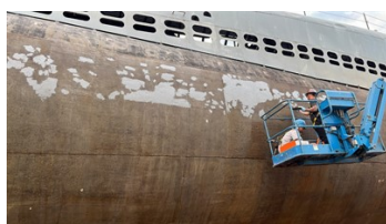
Contractors applying Belzona 1121 across the pitted waterline of the entire hull of the submarine.
