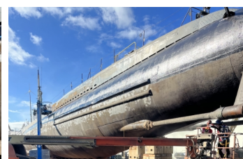
The hull of the submarine being painted over after the Belzona 1121 was fully applied and cured. Application finished.
