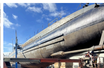
The hull of the submarine being painted over after the Belzona 1121 was fully applied and cured. Application finished.
