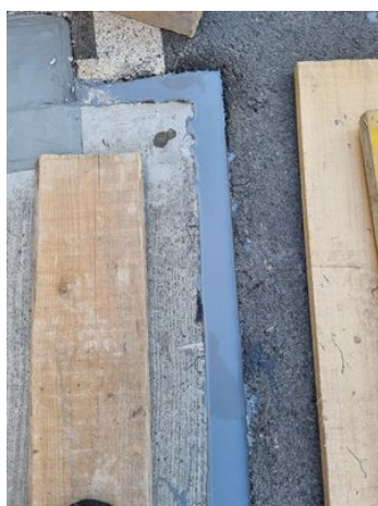
Belzona 4511 applied on sides and Belzona 4521 applied on the horizontal section of the joint.
