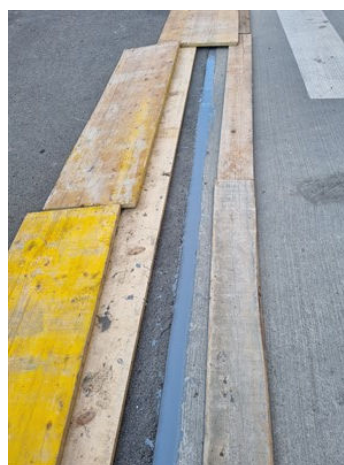
Installing thick planks after the application in order to enable traffic. We used those planks also during the application.
