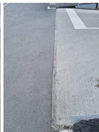
Situation after 7 months, with Belzona sealants still intact and in perfect condition.
