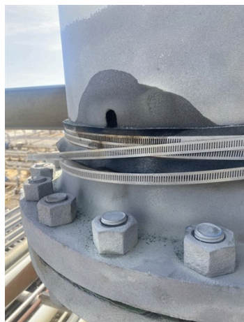
Line clamp leaking.
