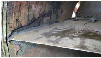
Damages to the valve's body.
