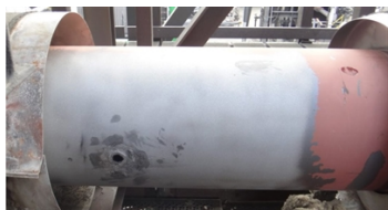
Defect in the pipe
