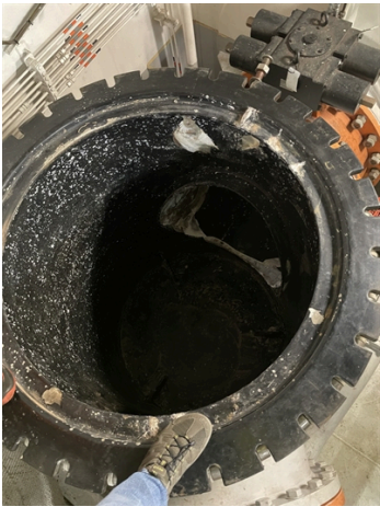
Flaking and damaged lining
