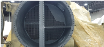
Overview of chiller
