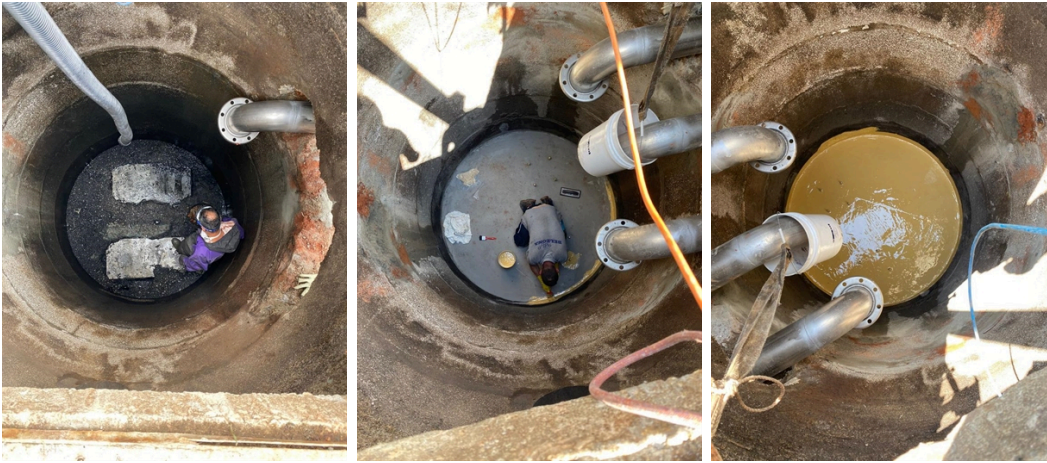
The damaged concrete area
