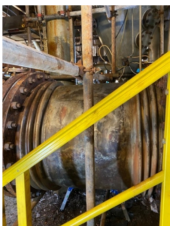
Worn and cracked bellows between two convolutions
