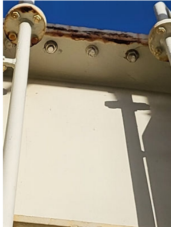
Typical corrosion at the main flange
