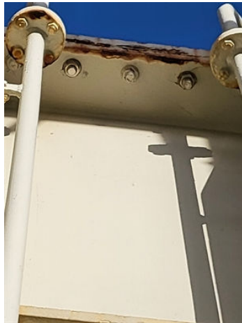
Typical corrosion at the main flange
