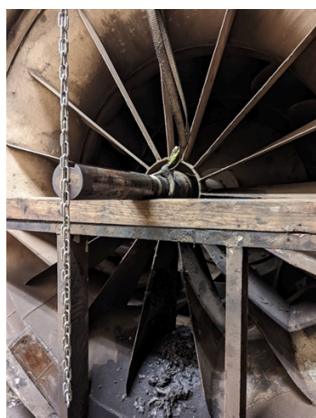
Air handler Unit
