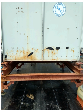
Damaged cooling tower
