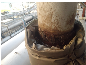
Corroded pipe section
