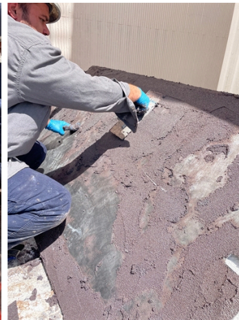
Belzona 1812 being applied to prepared plate to get ready to bond it to the chute.
