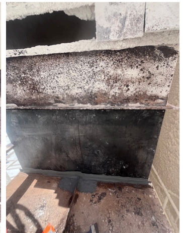
Job complete. Belzona 1212 and reinforcement cloth used to repair holes then a plate was boned with Belzona 1812 for abrasion protection.
