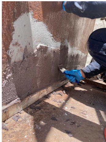
Area being prepared for application of Belzona 1212 and plate bond with Belzona 1812.
