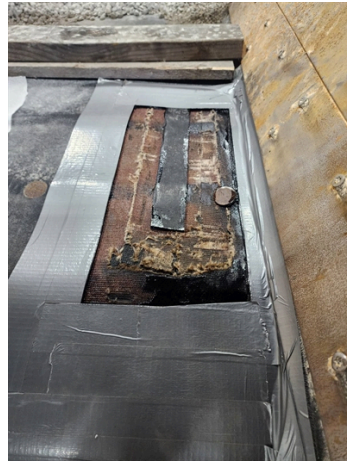
Top layer removed, Belzona 9341 reinforcement sheet pre-cut, border taped off, and Belzona 2911 QD conditioner applied.
