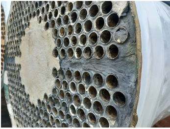
Condition of the faces upon arrival at the workshop
