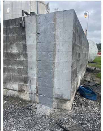
The crack in the outside of wall that was repaired with Belzona and coated
