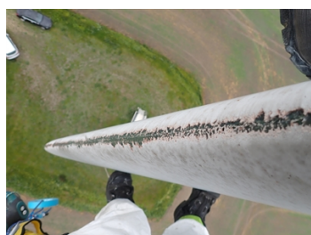
Damaged leading edge
