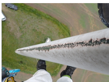
Damaged leading edge
