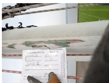
Wind turbine in need of repair and protection
