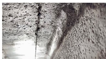
Example of the damaged surface of the application site.
