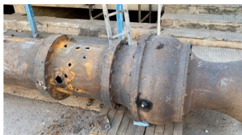
A damaged pipe with corrosion and through-wall holes.
