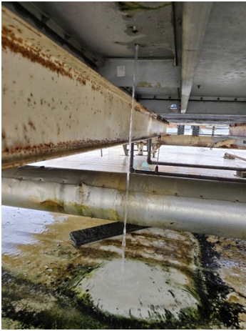
The constant stream of water leaking from the largest hole.
