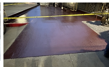
2nd and Final Coat of Belzona 4311 Applied Incorporating Aluminum Oxide for a nonskid finish
