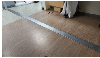
Aluminum cover plate causing bump and trip hazard
