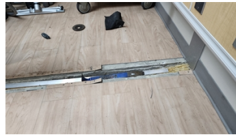
Plate removed and condition of underlying joint
