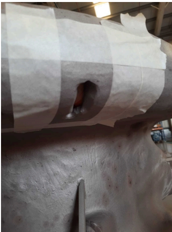
WIDENED CRACK LINE DRILLED ON BOTH ENDS.
