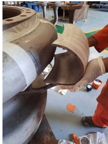
DRY FITTING OF THE PLATE PRIOR TO HOLE SEALING AND PLATE BONDING
