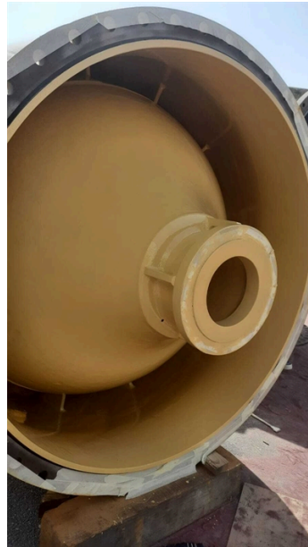
Application of first and second coat was completed and in this is the completed third coat application.
