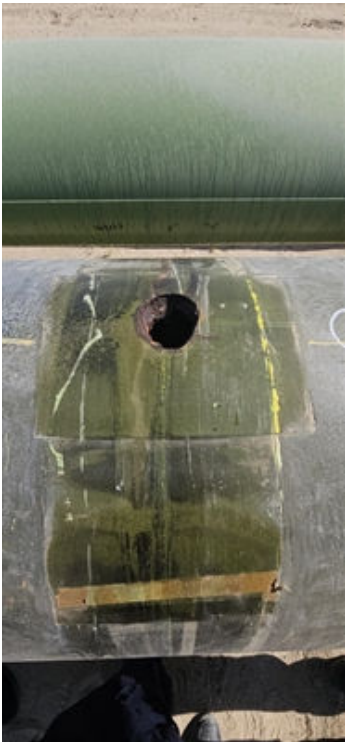
Pipe defect prior to Belzona application
