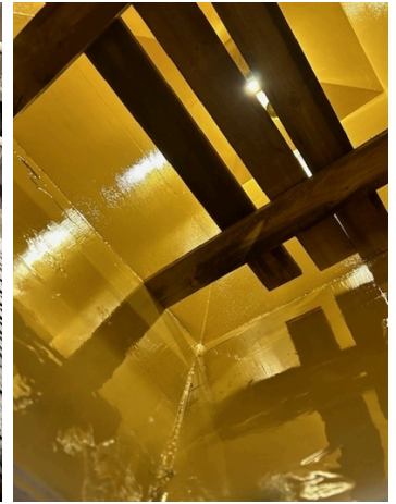
Platforms set up internally for applicators to stand on during the application process.
