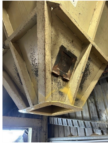
Tapered bottom end making bottom access difficult.
