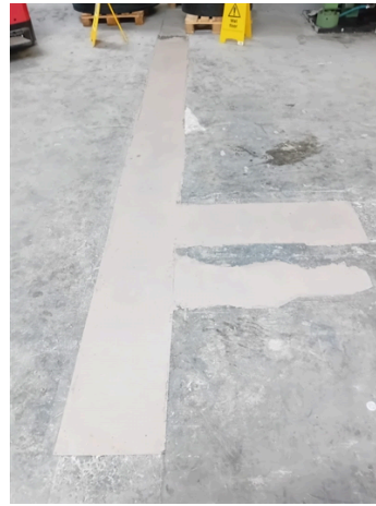
Damaged area fully repaired, screeded and feather edged with Belzona 4131 MagmaScreed to provide flat safe running surface for fork lift trucks and handling machinery
