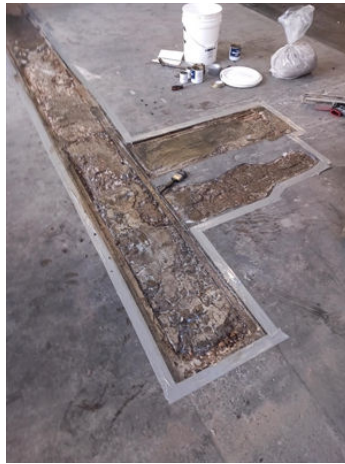
Damaged area prepared and conditioned with Belzona 4911 ready to accept Belzona 4131 MagmaScreed
