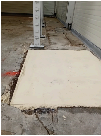
Uneven floor area made good using Belzona 4111 MagmaQuartz to support main racking stanchions
