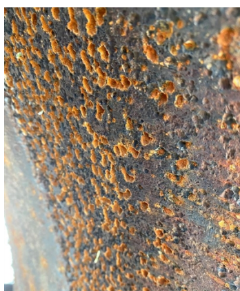
Closed-up look at the pits and damage of the nozzle
