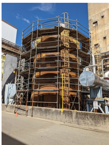
Tank experiencing corrosion.
