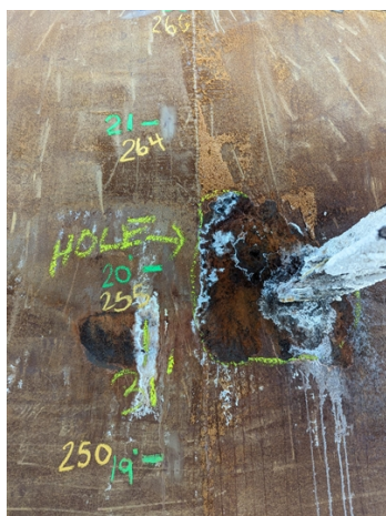
Close-up of corrosion.
